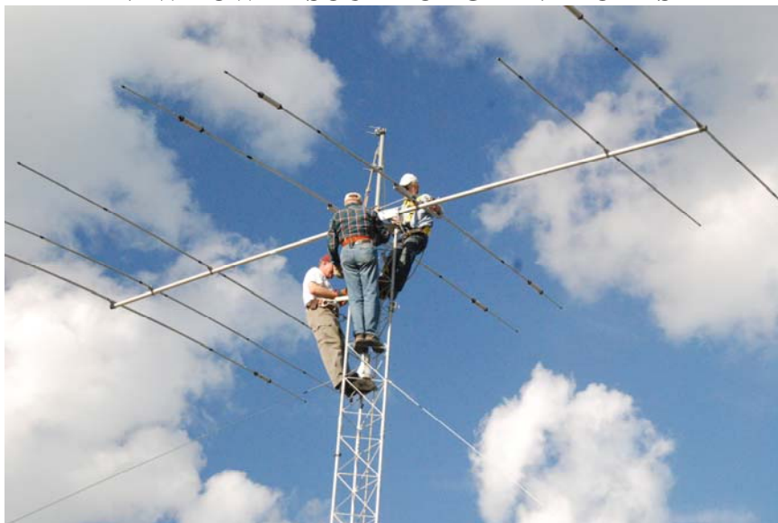
(l-r) Jim KC0XW, John KB0BSJ, Rod KE0A installing the HF Beam on Nancy KC0YXB's new tower (Photos by Nancy KC0YXB)
