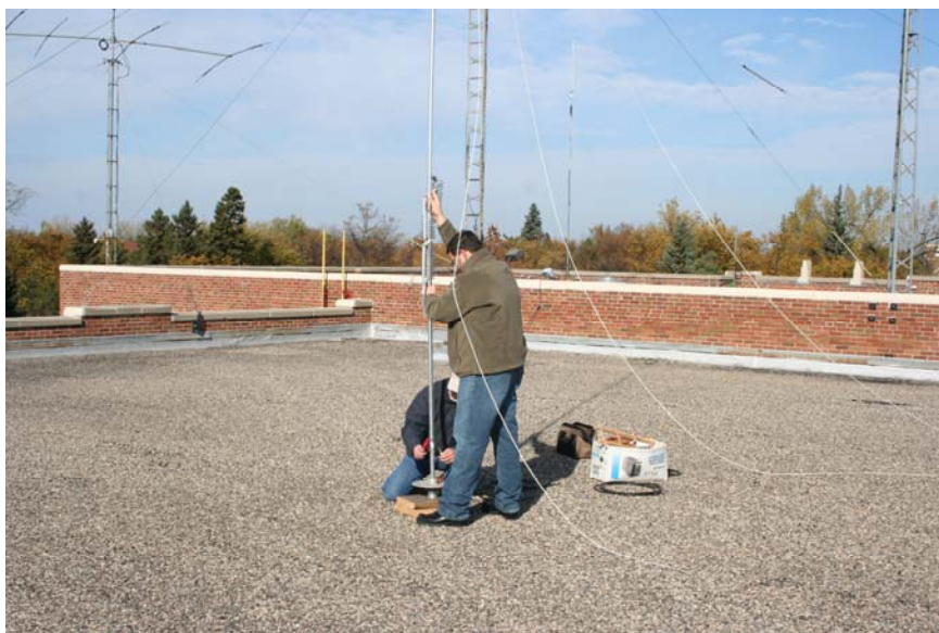
(l-r) Rod KE0A and Lance KC0YWZ installing a temporary vertical to be used for upcoming November Sweepstakes
